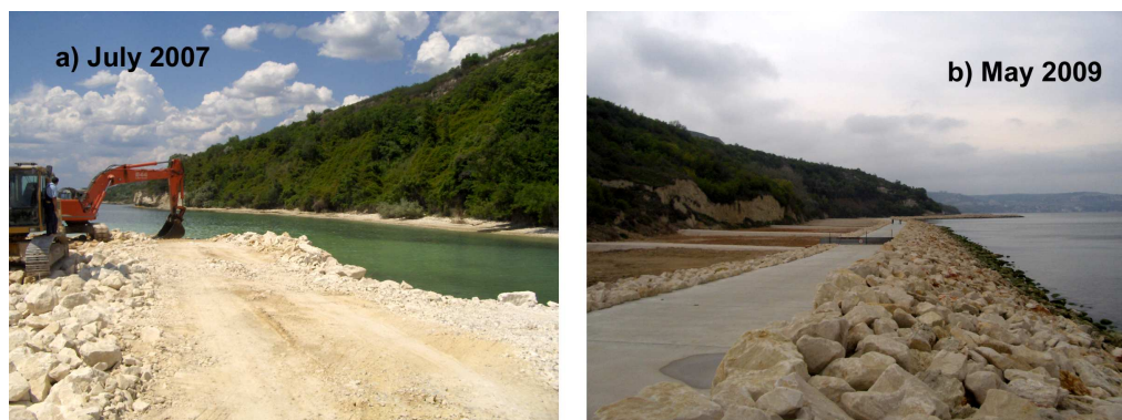
Fig. 4. Example of dike construction along the Bulgarian coast: a) June 2007; b) May 2009
